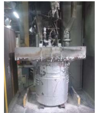
Figure 2: Customers previous ladle heater system
