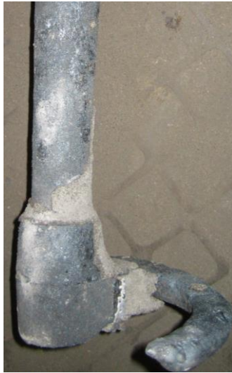
Figure 10: Frozen metal blocks the filter
